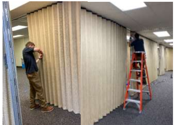
Service Specialists Jake and Jason from W.L. Hall did the early repairs
